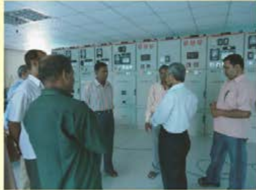
Visit to Patuakhali 33/11 KV Substation Cont. Room
